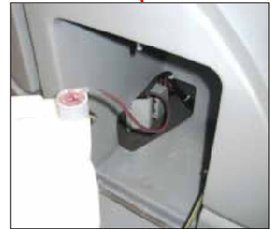
Detergent Pumps M10 and M11 (behind cover panel)
