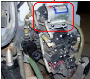
Mist Pump M5 and Solution Filter
