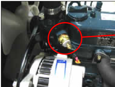
Coolant Temperature Sensor (above alternator)
